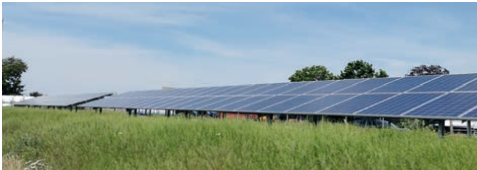
System power: 49 kWp
