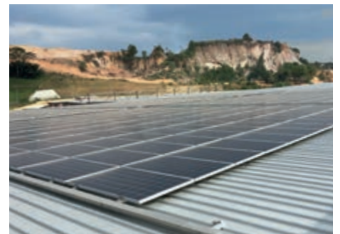
System power: 445 kWp
