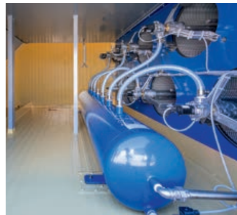
Filter cleaning with compressed air
