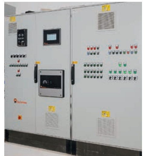
ViperTouch (integrated in the control cabinet) controls the system
