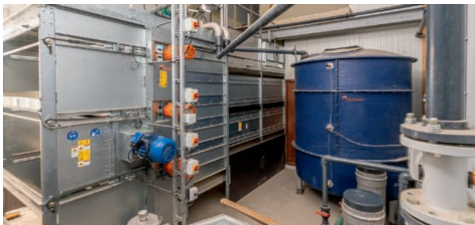
The liquid proportion is stored in a storage tank
