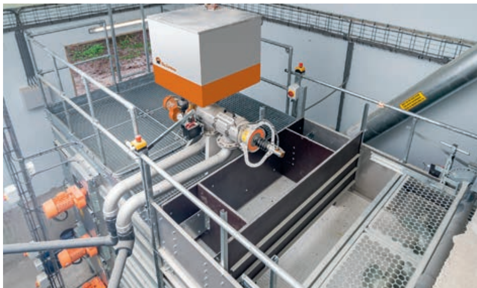
A screw press separates the untreated slurry into a solid and a liquid proportion
